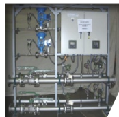
Water / Gas manifold
